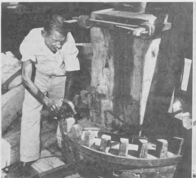
STURDY WOOD gears, left, probably part of the original mechanism, are re-installed by a workman. Evidence of the hand work that went into beams and gears can be seen at right.
